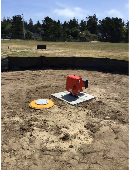
Runway 33 REIL Unit
