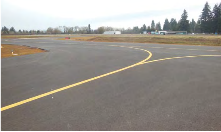
Below: Scappoose taxiway project Right: Scappoose taxiway lighting
