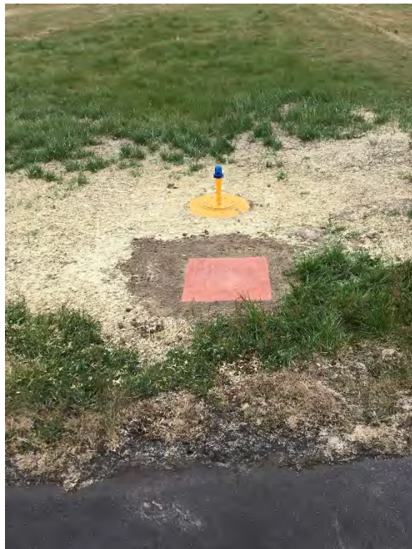
Duct Bank Marker
