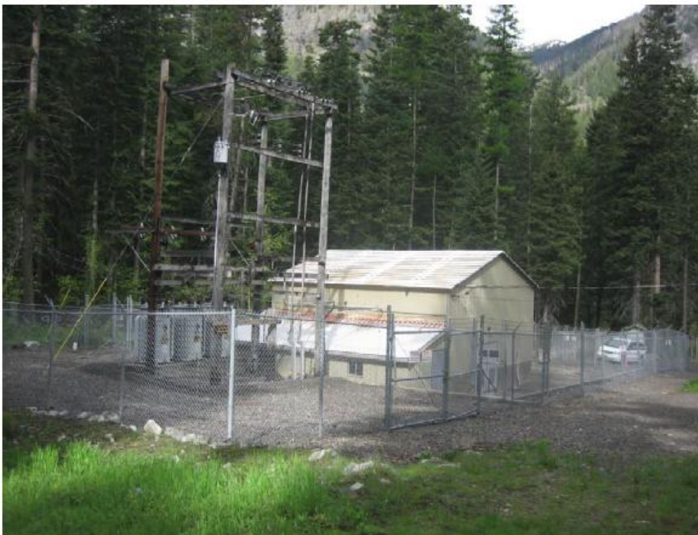
Figure 11: Project Powerhouse and switchyard with transformers. (PacifiCorp, 2011)
