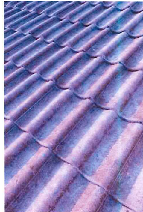
Old purple corrugated asbestos cement roof sheet.
