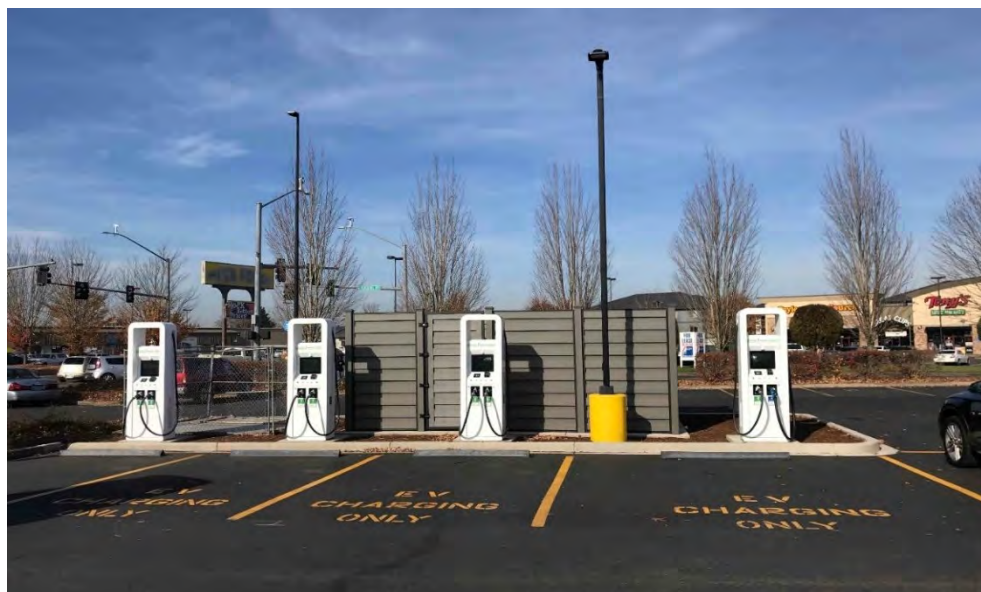
Electrify America Charging Station in Salem, Oregon with Extra-Wide Clearance for Accessibility. Source: Electrify America
