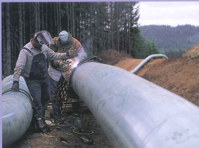
Contract welders make tie-in welds to connect sections of the 24-inch diameter pipe that was laid underground for the 1999 Mist gas storage expansion project.
