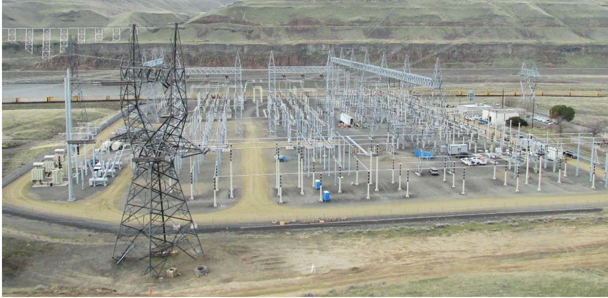
Figure B-25. Typical 500-kV Station
