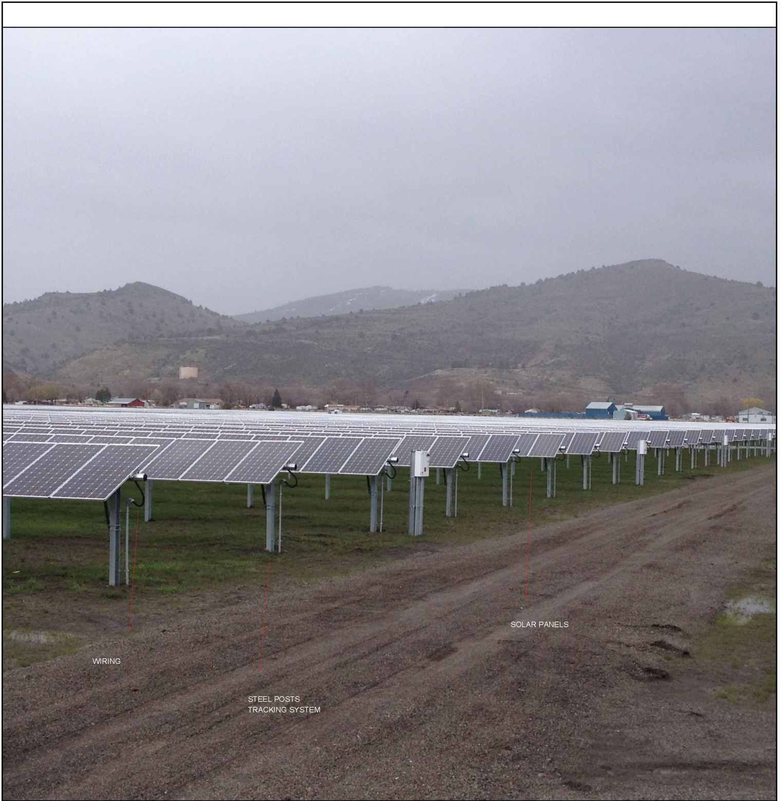
Figure B-5 Illustration of Installed Solar Facility
