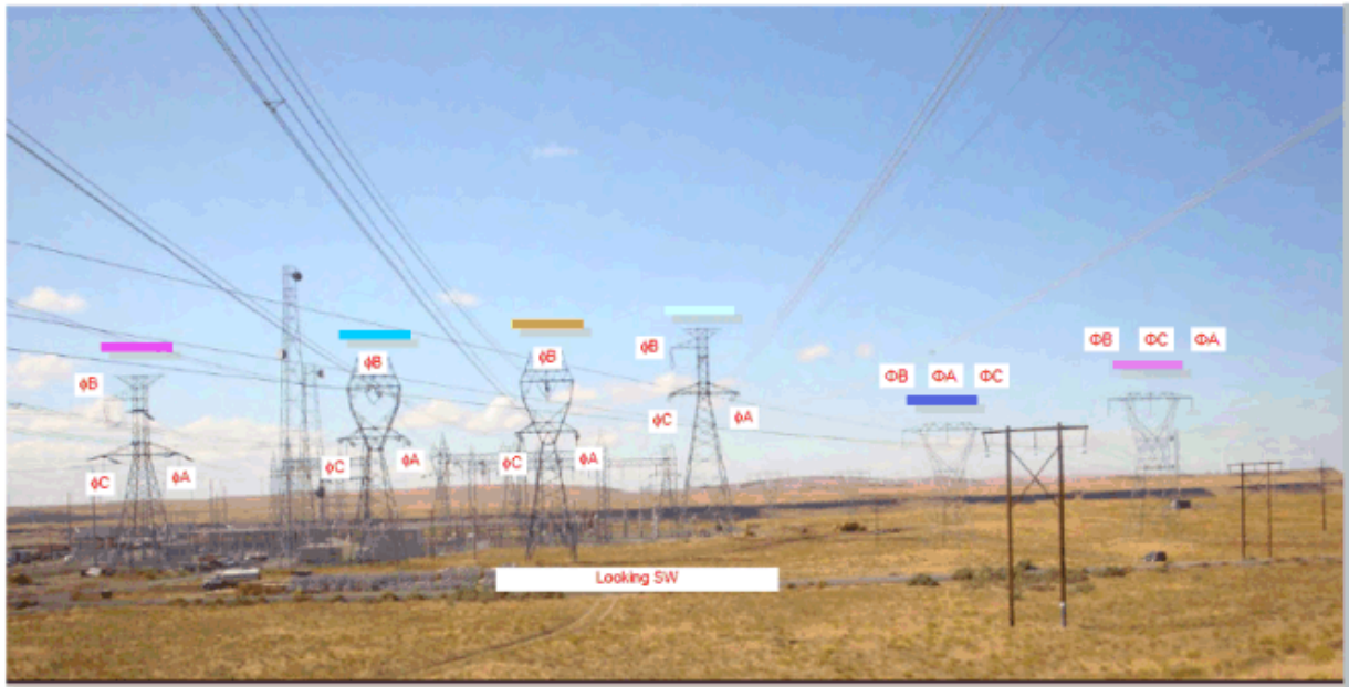
Figure 12 - Photo of Existing Line Configuration at Slatt Substation Joint Corridor ROW
