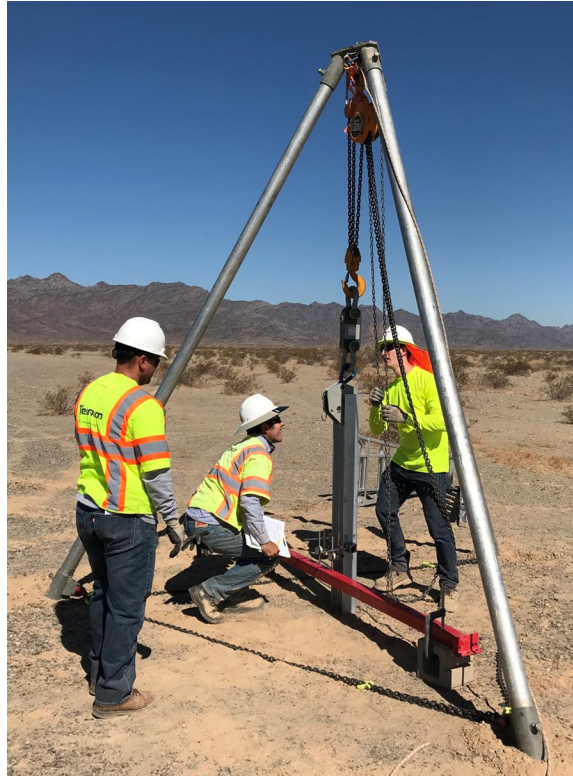
Typical Photo of Tripod with Chain Fall, Load Cell, and Dial Gauges.
