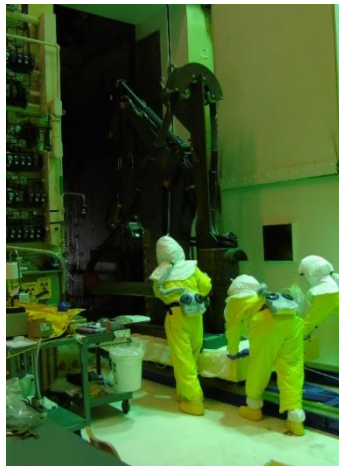
Following testing and training in a mock-up, crews install first remote excavator
