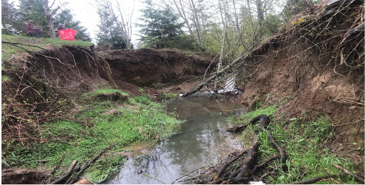
Exhibit A: Unnamed tributary in King City Community Park. Erosion is the result of unmitigated stormwater runoff from the uphill Bull Mountain community. The headcutting of this stream is occurring at a rate of approximately 8 feet per year.
