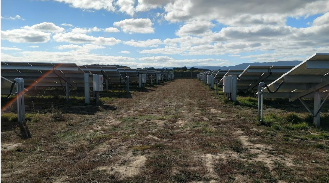
Figure 56. Oregon Solar Farm, Willamette Valley
