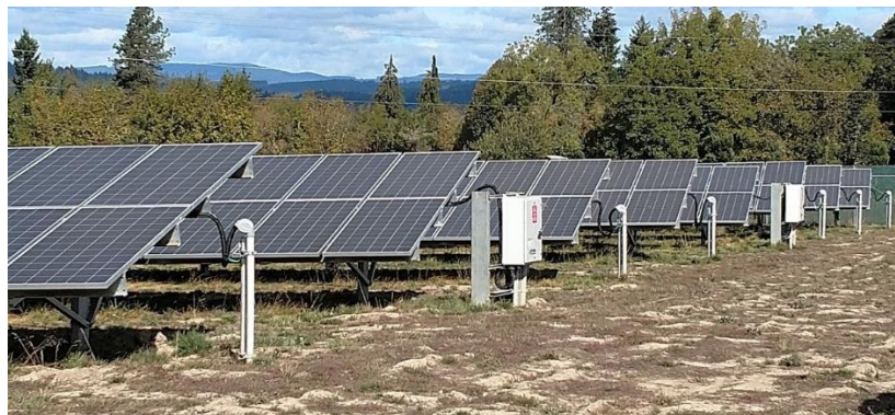
Figure 49. Oregon Solar Farm, Willamette Valley
