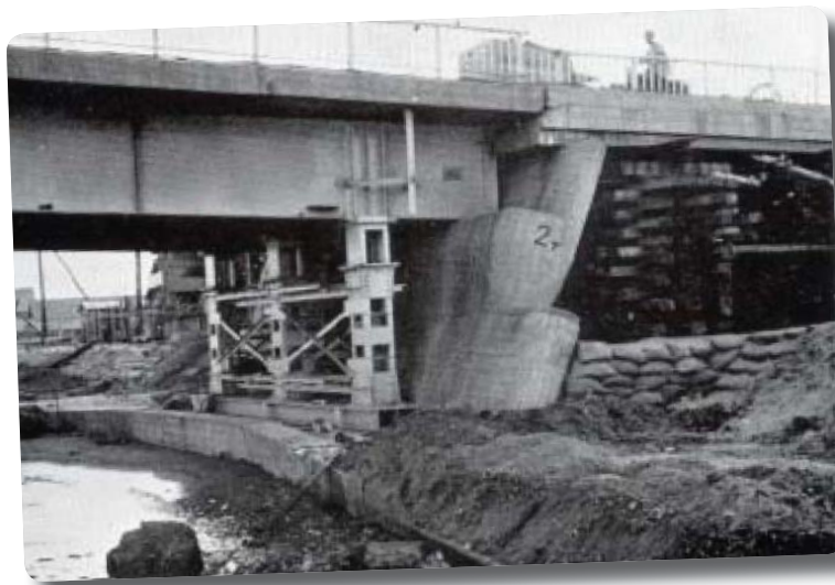
Figure 2.1 : Bridge pier damage resulting from liquefaction and lateral displacement of foundation soils (Yachiyo Bridge, 1964 Niigata, Japan)
