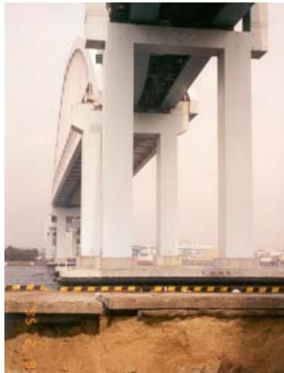
Figure 2.31: Displacements to Bridge Foundations at Rokko Ohashi Bridge
