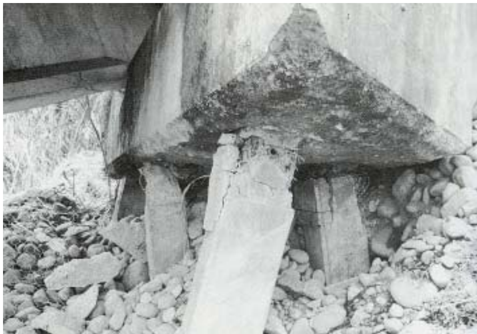
Figure 2.25: Rio Vizcaya Bridge, Pile Failures (North Abutment)
