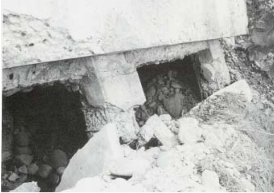
Figure 2.26: Damage due to Liquefaction at Rio Banano Bridge
