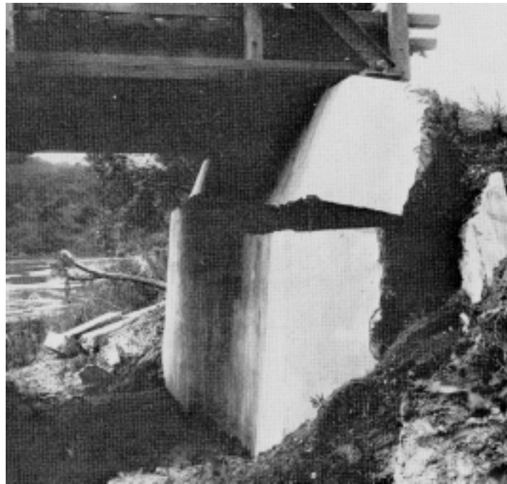
Figure 2.1: Pajaro River Bridge Damage
