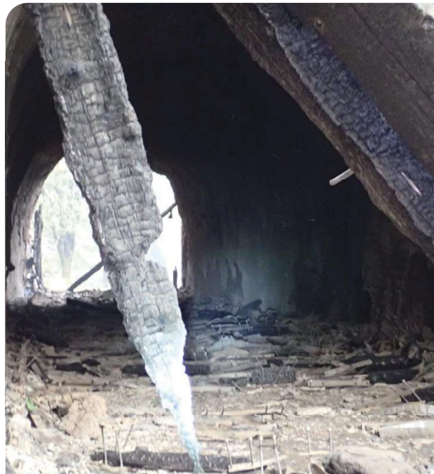
Oneonta Tunnel after 2017 Eagle Creek Fire.
