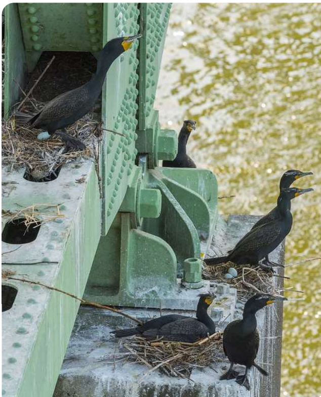
Cormorants nesting on the Astoria-Megler Bridge add salt-rich waste to the surface, accelerating corrosion. Photo by ODOT Photo Video Services.
