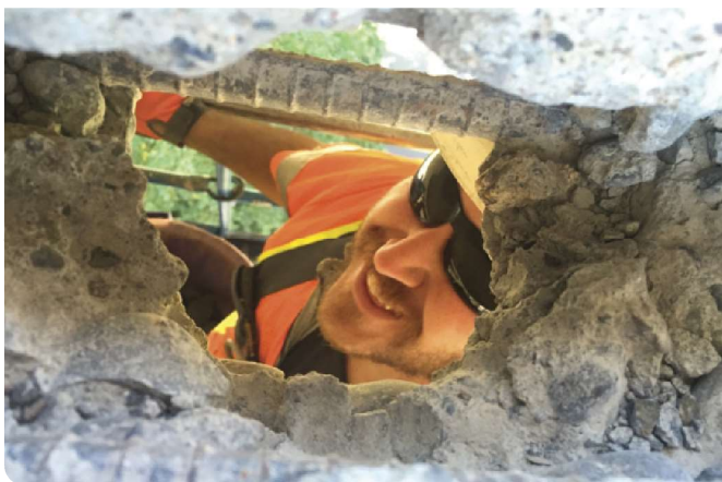
The hole developed on a Fremont Bridge ramp. Full depth deck failure of the roadway can be expensive for both maintenance and replacement. Photograph by Jeremy Kappers
