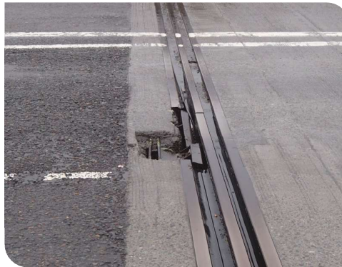
Damaged Bridge Joint.
