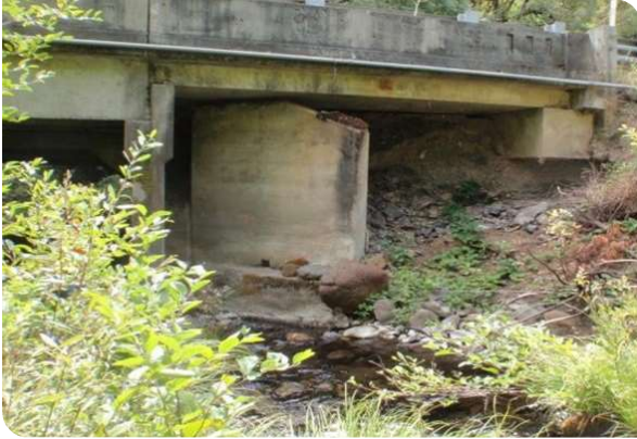
Substructure deterioration can include damage from high water events and can result in the need to replace the bridge.
