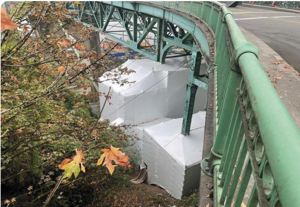
An ODOT contractor constructed a containment on the west end of the St. John's Bridge to access the concrete piers. When damaged concrete is widespread on a big bridge, concrete repairs can rise from maintenance to preservation work. Photo by Mats Halvardson.
