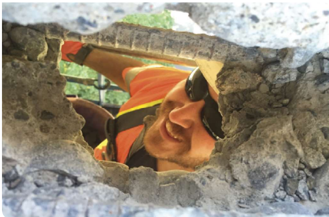
The hole developed on a Fremont Bridge ramp. Full depth deck failure of the roadway can be expensive for both maintenance and replacement. Photograph by Jeremy Kappers, Region 1 Bridge Maintenance Specialist.
