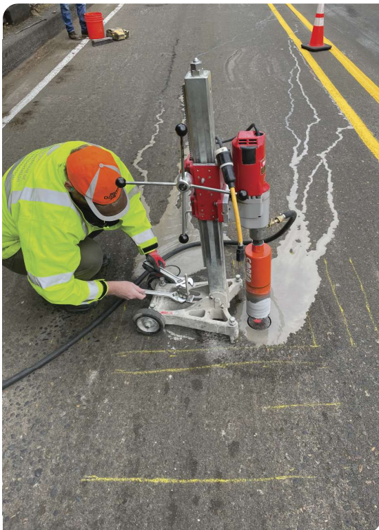
Coring a bridge deck to determine chloride levels. This enables better decision-making for future overlays. Photo by James Garrard.
