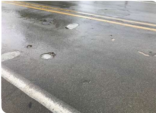
Deck deterioration can include cracking, scaling and surface spalling which result in safety concerns, and increased wear and tear on vehicles that use the bridge.
