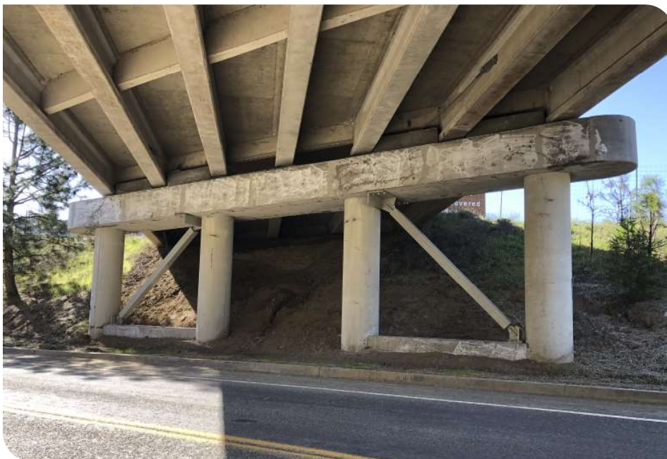
Bent strengthening using buckling restraint bracing (BRB) on Southern Oregon Seismic Bridge Retrofit Project. Photo by Bob Grubbs
