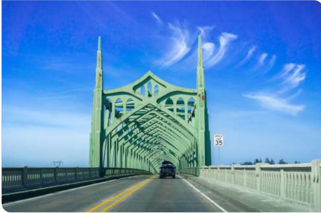
Coos Bay Bridge, coastal bridges are particularly susceptible to accelerated corrosion from airborne oceanic salts and wildlife waste deposits that contain salts.
