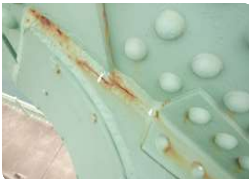
Superstructure deterioration can include corrosion, cracking, and fatigue damage for steel bridges.
