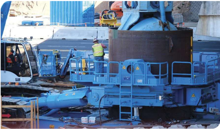
Oscar the oscillator, largest of its kind put in to action for seismic retrofit of the Abernethy Bridge.
