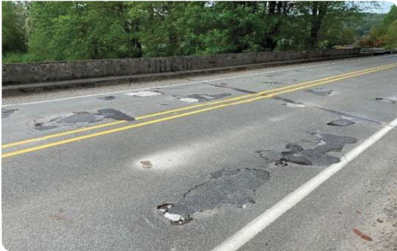
2. Percent of NHS bridges by deck area classified as in poor condition
