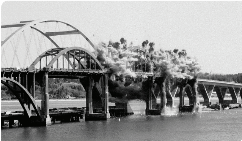
The demolition of the Alsea Bay Bridge in 1991. The replacement bridge is in the background.
