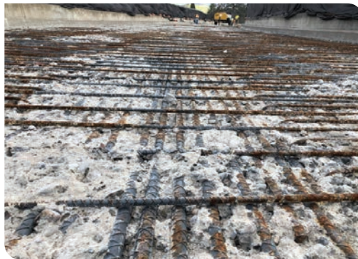
Deck deterioration can include cracking, scaling and surface spalling which results in safety concerns and increased wear and tear on vehicles that use the bridge.
