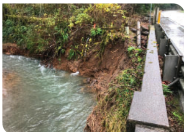
Seasonal scour damage.
