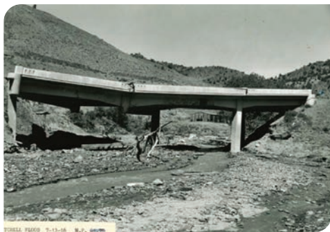
The Bridge Creek Bridge on Oregon 41 was built in 1953 and failed due to scour after major flooding in 1956. This bridge, while relatively new, was not able to withstand the erosive forces of extreme water velocity and debris flow and the resultant scouring of embankments and bridge foundations.
