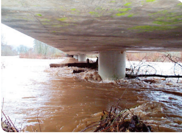
Substructure deterioration can include damage from high water events and can result in the need to replace the bridge.
