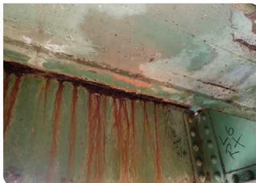
Superstructure deterioration can include corrosion, cracking, and fatigue damage for steel bridges.
