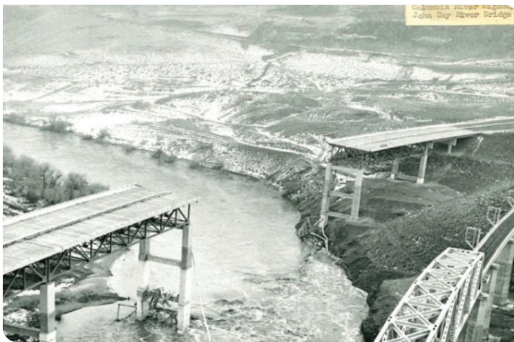
The John Day River Bridge on I-84 was newly built in 1963. The next year, following a series of extreme storm events, the bridge failed due to scour surrounding one of the piers. The pier eventually washed away taking a portion of the bridge with it.
