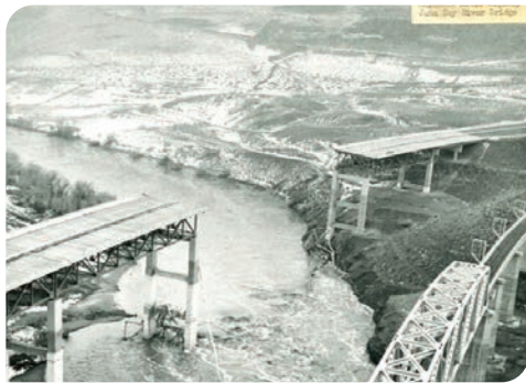
The John Day River Bridge on I-84 was newly built in 1963. The next year, following a series of extreme storm events, the bridge failed due to scour surrounding one of the piers. The pier eventually washed away taking a portion of the bridge with it.
