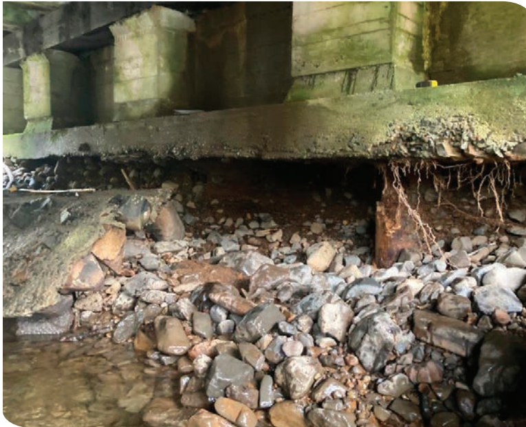
Scour problem threatening the bridge structure.
