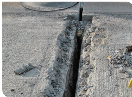
Damaged bridge joint.
