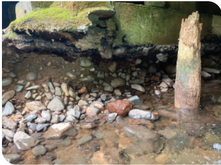
Many years of scour activity weakened the foundation support.
