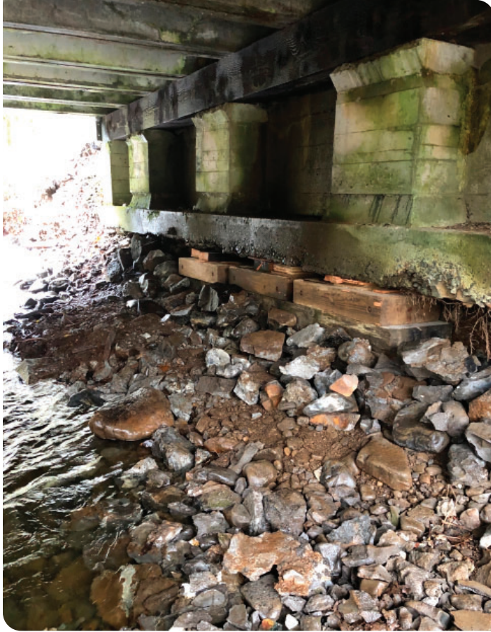
Temporary support provided as part of the emergency repair to prevent catastrophic failure.
