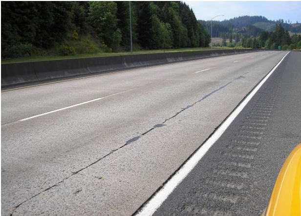
High – right wheel path (based on width and spalling)
