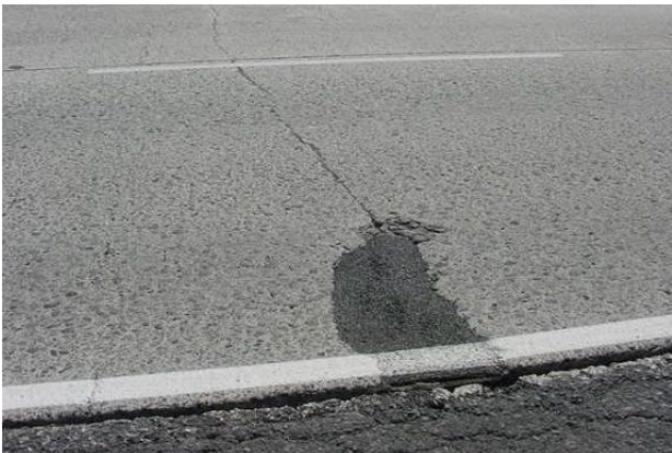
High severity punchout covered with high severity patch
