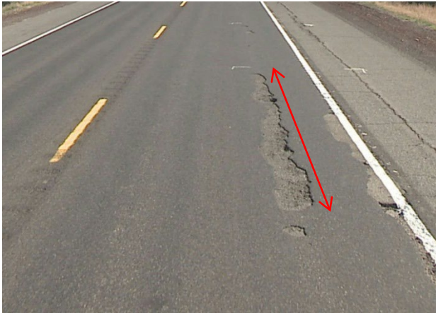
Low severity – count as two potholes (continuous shallow pothole is 25' long)
