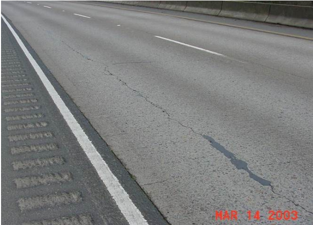
Low – left wheel path (sealed crack)
