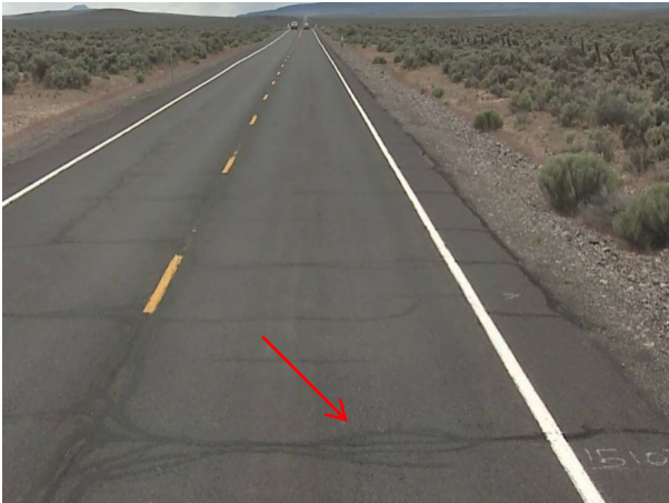
Moderate severity (due to adjacent low severity cracks)
