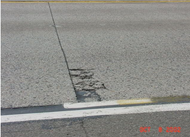
High – faulted over 1/2”
