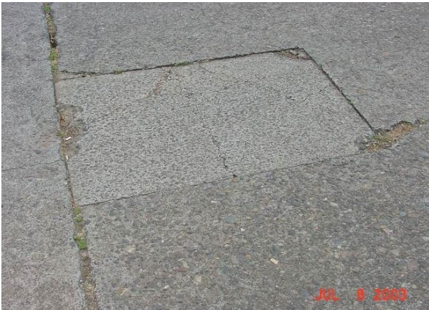
Moderate – patch displays faulting < 0.25"
