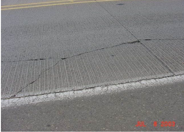
Moderate – crack has low severity (< 3” wide) spalling for > 10% of length
