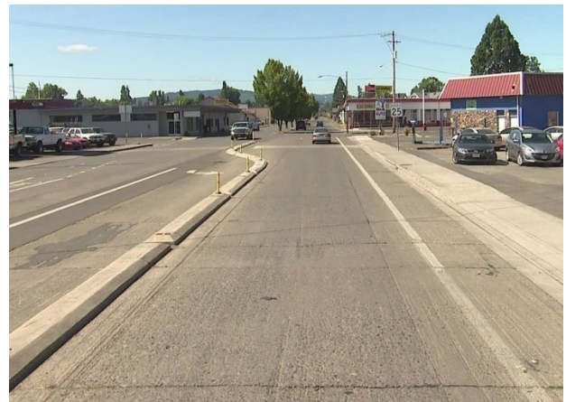
Uneven surface grooves are not rated as longitudinal cracking.
