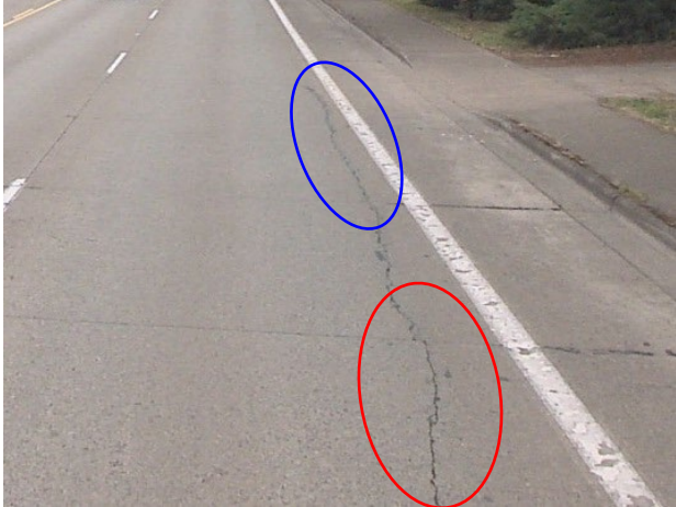
Right wheel path – low severity (red circle) becomes right edge – low severity (blue circle)
