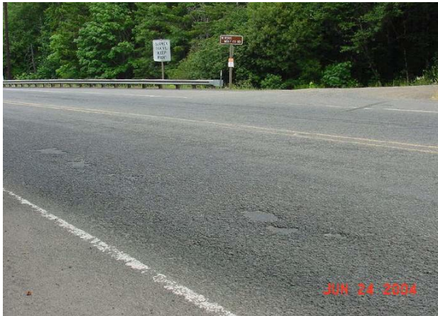
High (with potholes)
