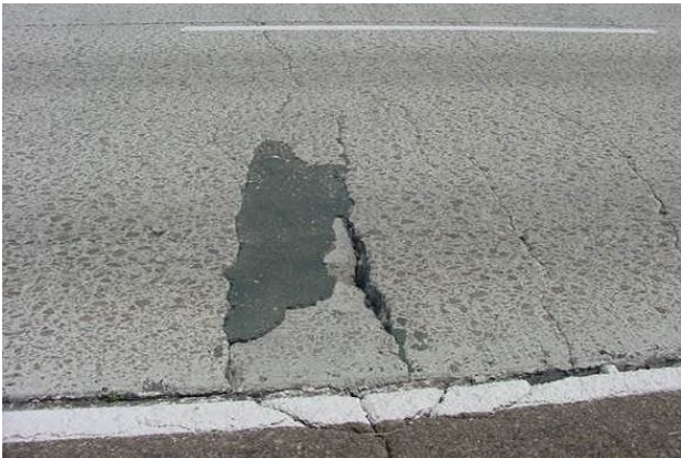
High – more than 0.5” faulting
