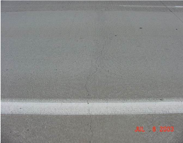
Low – transverse crack width < 0.125", no faulting or spalling
