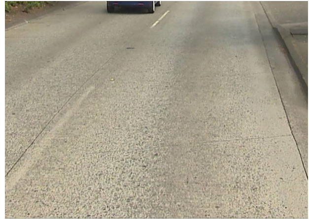
Worn surface may have barely visible hairline cracking, which is not rated.
