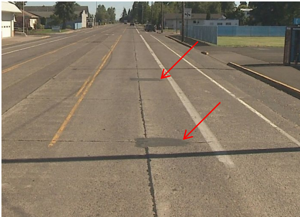
Moderate – small irregular-shaped asphalt concrete patches
