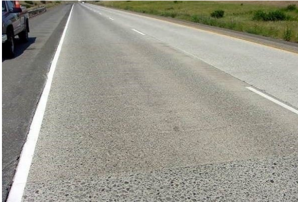
Low severity patch, note tight T-cracks
