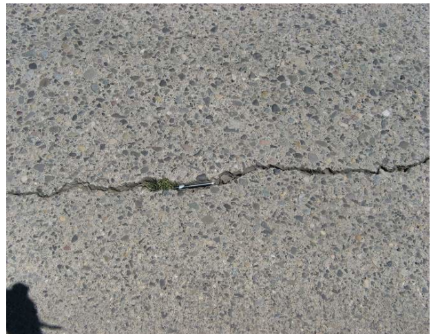
Up close picture of the crack
