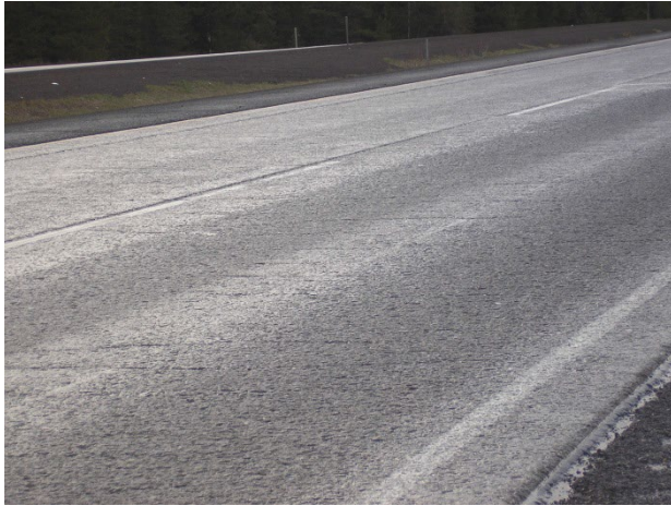
Rough surface may have barely visible longitudinal cracks that should not be rated.
