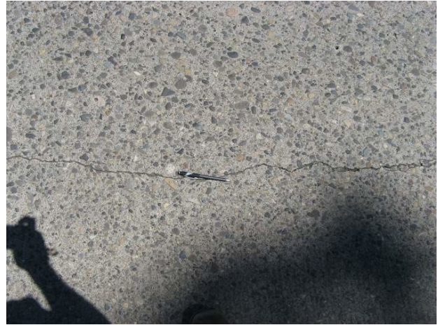
Up close picture of the crack
