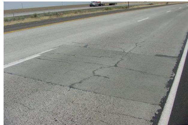
Moderate – patch has moderate longitudinal cracks
