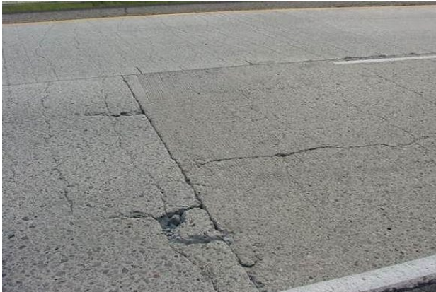
Moderate – spalling between 3” and 6”
