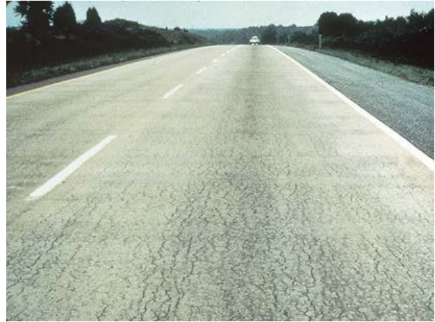
Do not rate map cracking (image from LTPP Distress Identification Manual).
