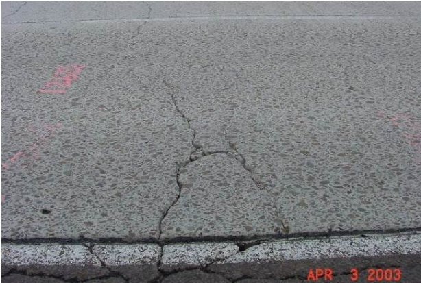
Moderate severity punchout – “Y”-crack with > 10% spalling in the branches
