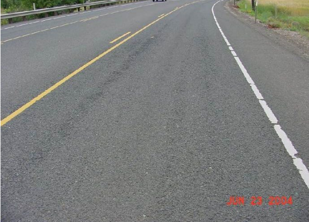
Moderate (in left wheel path) and low (in right wheel path)
