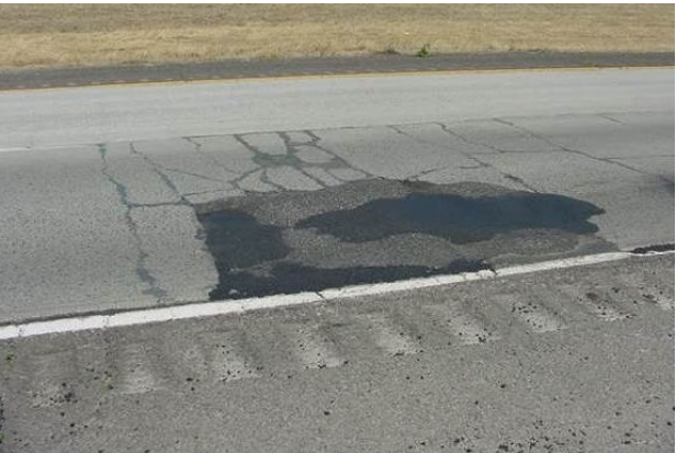
Multiple high severity punchouts covered with high severity patch, this is localized within a single area
