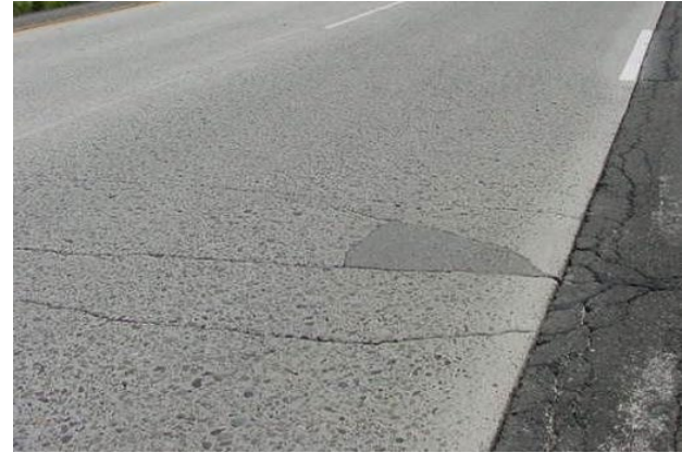
Moderate – irregular concrete patch completely repairing a punchout; record as patch not punchout
