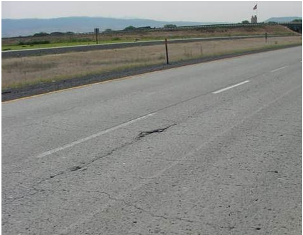
High – left edge (based on width and spalling)
