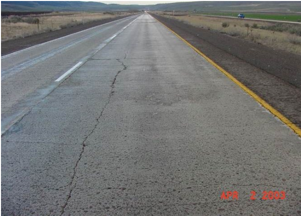
Moderate – left wheel path (due to spalling)
