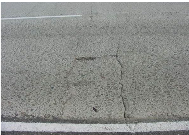
Low – spalling on T-crack and L-crack (if faulted over 0.25", rate as moderate)
