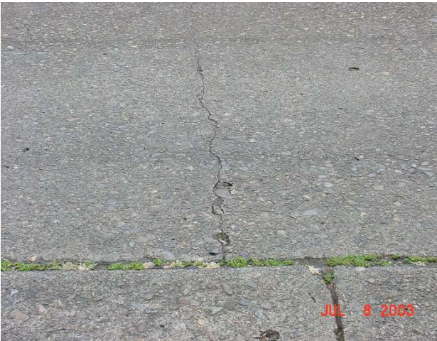
Moderate – transverse crack has spalling
