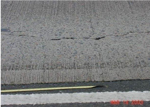
Not a punchout, spalling on L-crack only
