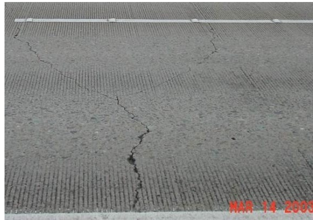
"Y"-crack – do not record as a punchout since branches are not exhibiting spalling, only the trunk is spalling
