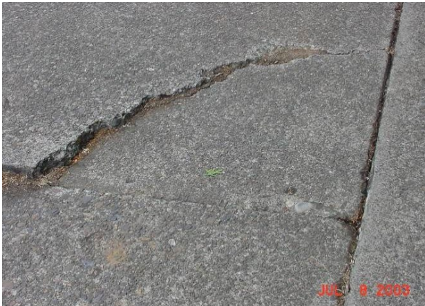
High – corner break broken into two or more pieces
