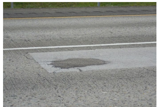
High – patch has high severity distress and additional patch material
