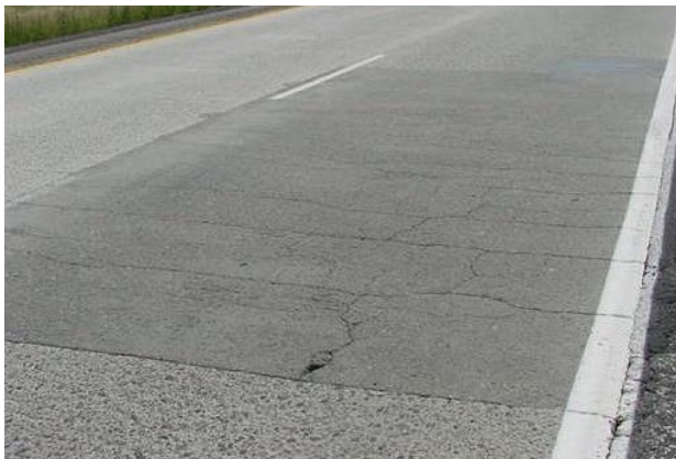
Moderate – patch has longitudinal crack with spalling
