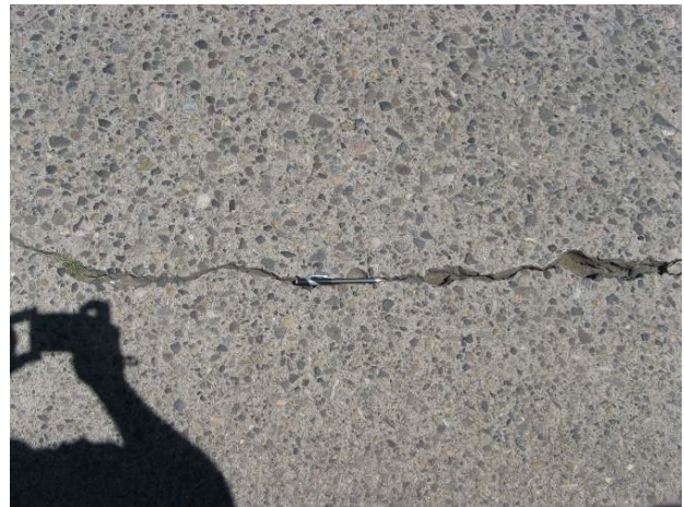
Up close picture of the crack
