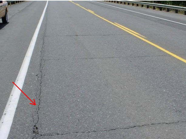
Left edge – moderate severity (low severity with adjacent random cracking)
