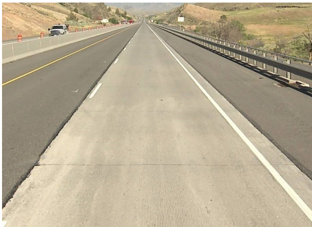
Longitudinal tining is not rated as longitudinal cracking.
