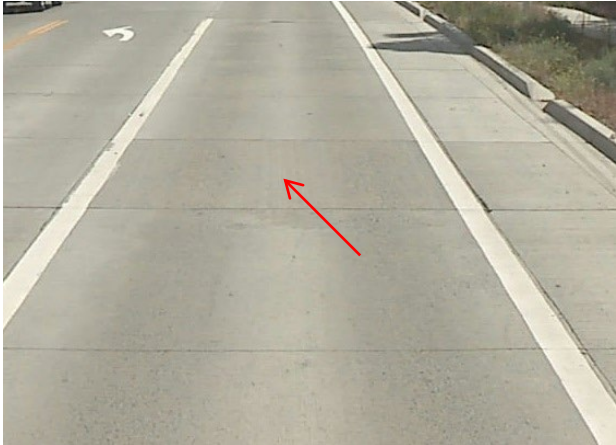
Low – patch has no distress
