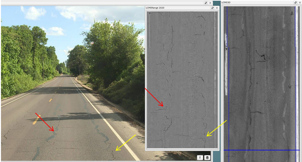
Sealed but open (red arrows) and unsealed (yellow arrows) longitudinal wheel path cracks.
