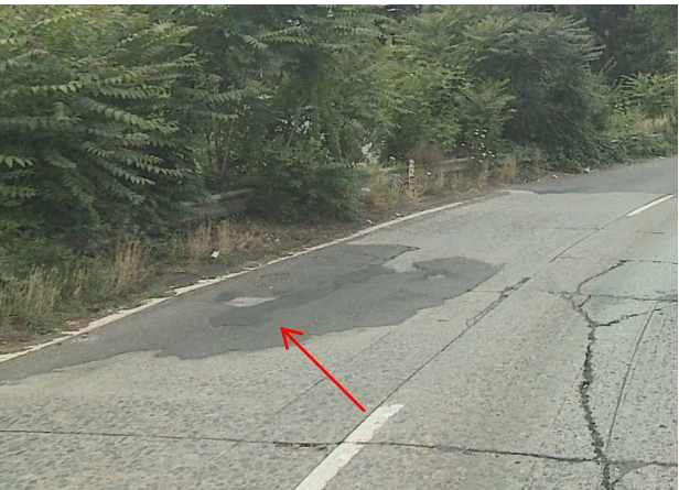
High – patch is severely deteriorated
