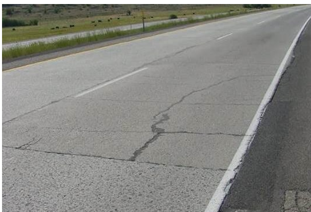
High – patch has spalled transverse and moderate/high severity longitudinal cracks
