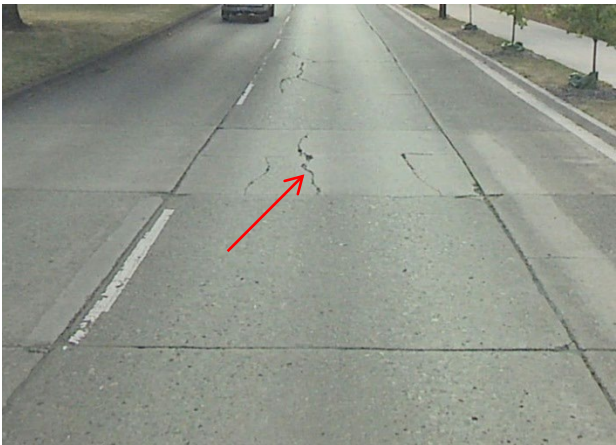
High – patch has high severity distress
