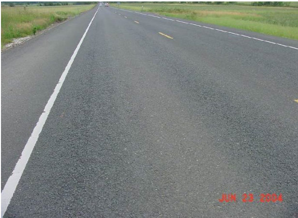
Low in wheel paths (open graded surface)
