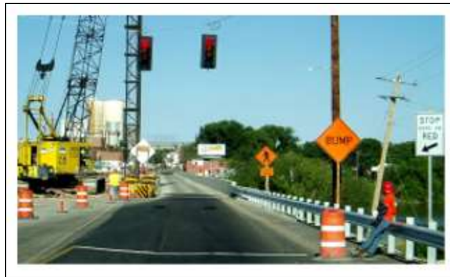
Figure 2-22: Temporary Traffic Signal (Span Wire)
