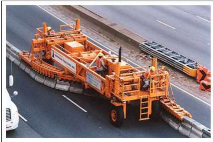
Figure 2-19: Concrete “Zipper” Barrier
