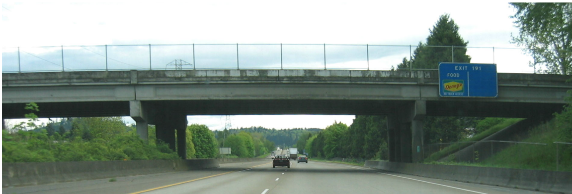
Figure 1.19. Typical Pre-cast I-Beam Overpass, Interstate 5, Lane County, OR Source: Author Photograph, May 2002
