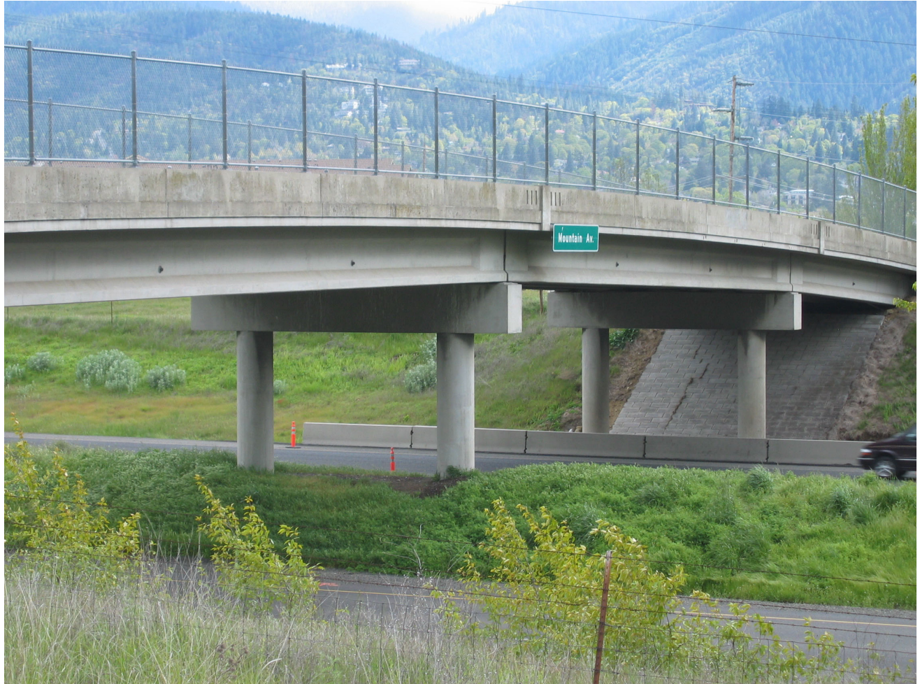
BRIDGE No. 8739, MOUNTAIN AVE OVER INTERSTATE 5, ASHLAND, JACKSON COUNTY OREGON, LOOKING SOUTH 259-Foot long Precast Concrete Girders (1963) with Type A/B Bridge Rail, Modified with Protective Fencing June 2003
