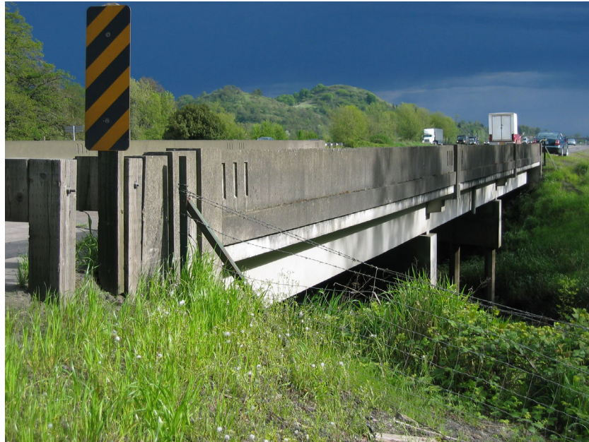
Figure 2.8. Type A/B Bridge Replacement Rail Isaac Constant Bridge, Central Point, Oregon Source: Author Photograph, November 2002
