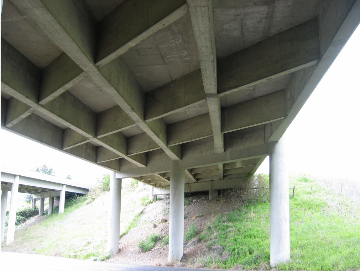
Figure 2.27. Round Section Piers, Bridge No. 8738N Interstate 5 over Eagle Mill Road, Jackson Cty, 1962 Source: Author Photograph, May 2002
