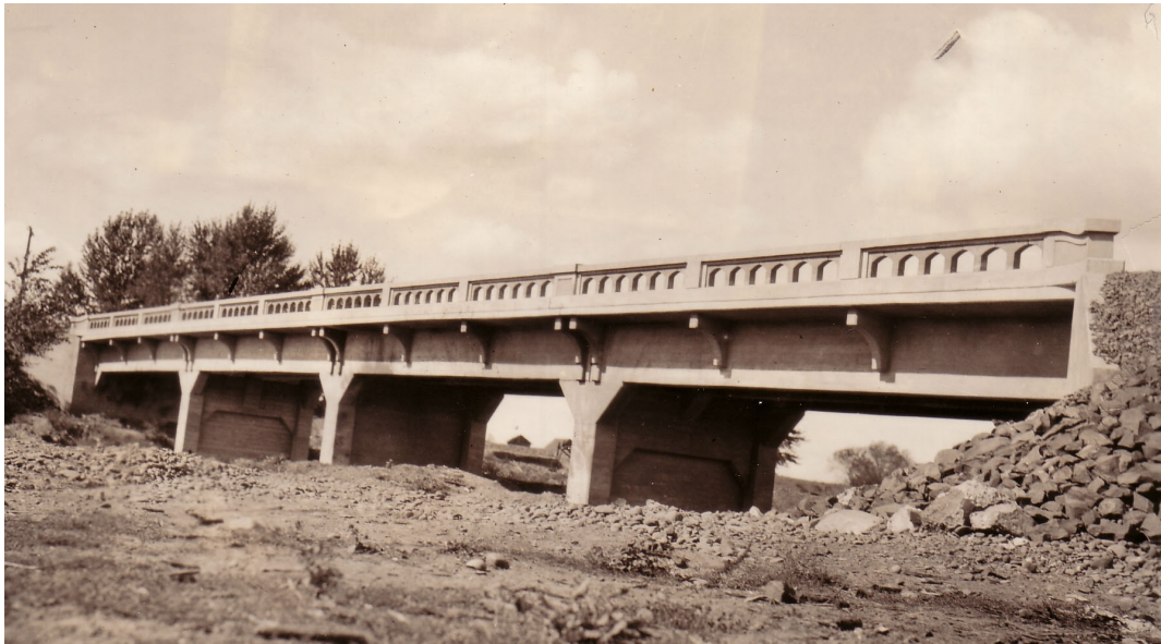
Figure 2.18. Standard Cast-in-Place Design, Umatilla River Bridge at Echo, Umatilla County, Bridge #1165, Built 1926 Source: ODOT Archive
