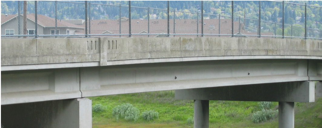
Figure 2.22. Typical Pre-Cast I-Beam with “Panel” Sides, Mountain Ave Overpass, I-5 Jackson County, Bridge #8739, 1963 Source: Author Photograph, May 2003
