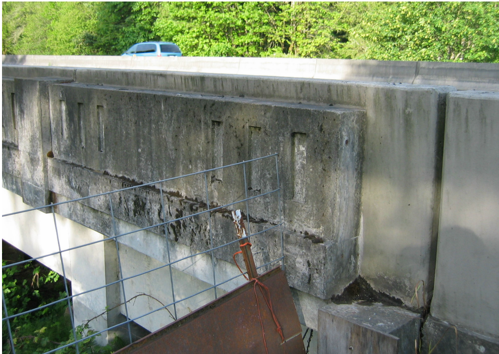
Figure 2.16. Type A Rail, Retrofit Bridge No. 7572A, Curtis Creek Bridge/I-5, Douglas County Source: Author Photograph, May 2003
