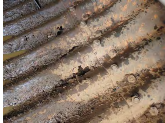
Rusted invert and voids under the culvert (9/20/16)
