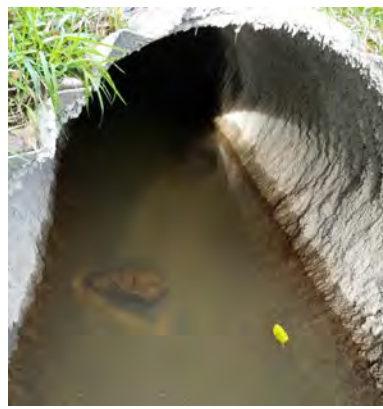
Outlet of culvert is backwatered
