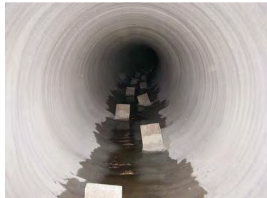
Inside culvert showing centrifugally cast concrete liner and simulated fish rocks
