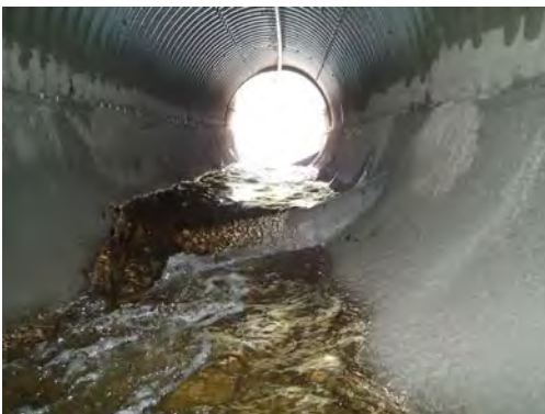
The slump in the middle of the pipe resulted in a less backwater at this weir location (near inlet) than anticipated (10/26/16)
