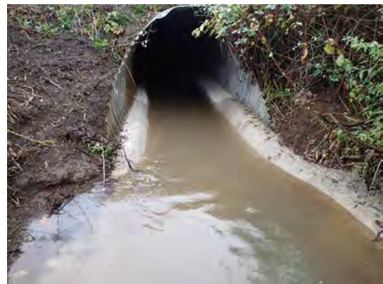
Culvert outlet – backwatered (10/26/16)
