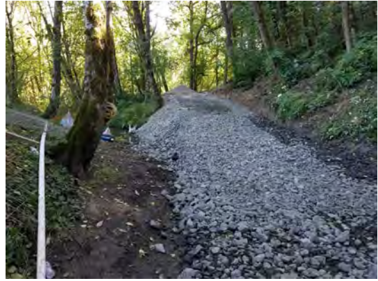
Access road at outlet - 2017. Water is piped around work area in pipe on right of photo
