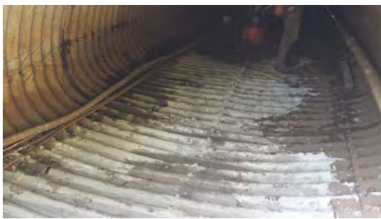
Grouting the invert to fill voids under the invert and reinforce the floor so that the fish rocks and invert paving can be installed (9/21/16)
