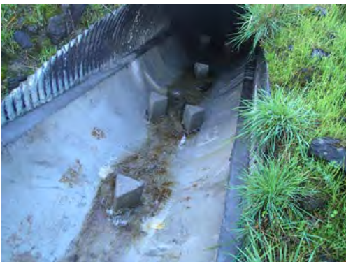
Roughness features creating turbulence, increased water depth, and longer flow path during low flow (10/26/16)
