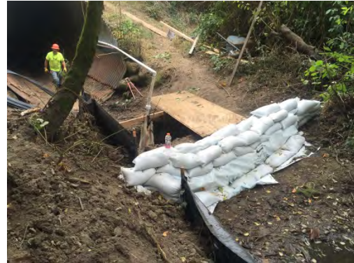
Work area isolation. The stream was not running but there were isolated pools in the channel (10/4/16)
