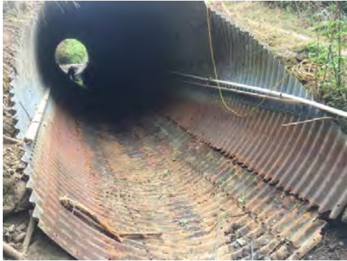
Rusted invert during construction, after the work area is isolated and culvert invert was cleaned out (10/4/16)
