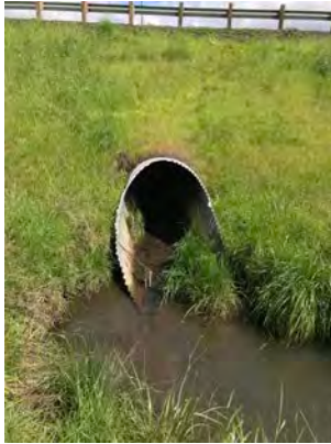
Culvert outlet before repair
