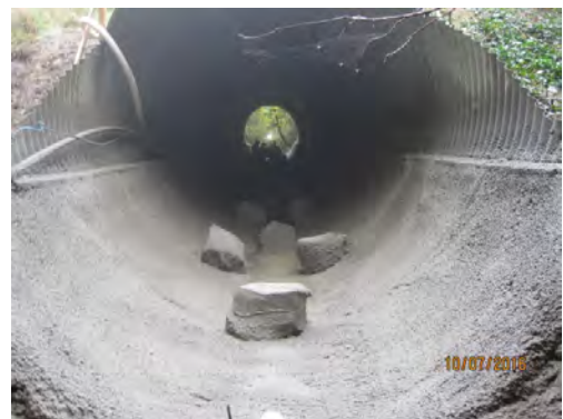
During invert paving - rocks are covered in plastic to keep the concrete off the natural rock surface (10/7/16)
