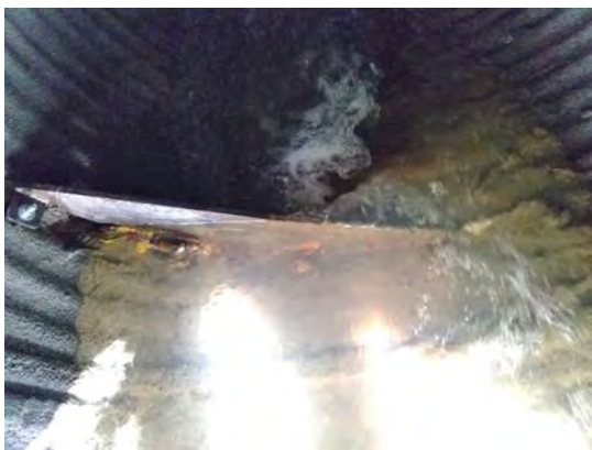
Baffle inside culvert showing resting habitat and deeper water
