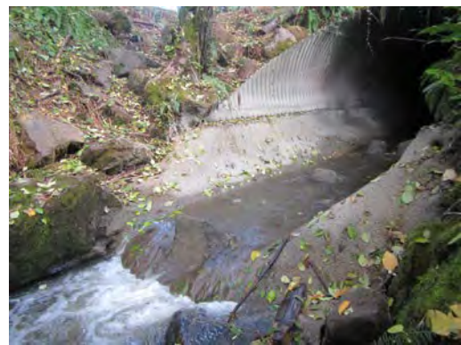
Culvert outlet at winter base flow. There is a steep section at the end of the culvert treatment - 2017
