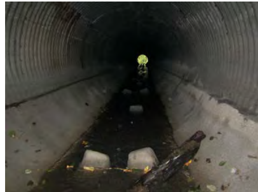
Inside culvert showing invert paving and simulated fish rocks – some debris on double rock installation
