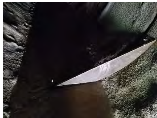
Baffle inside culvert during lower flow – steel corner baffles are bolted to culvert
