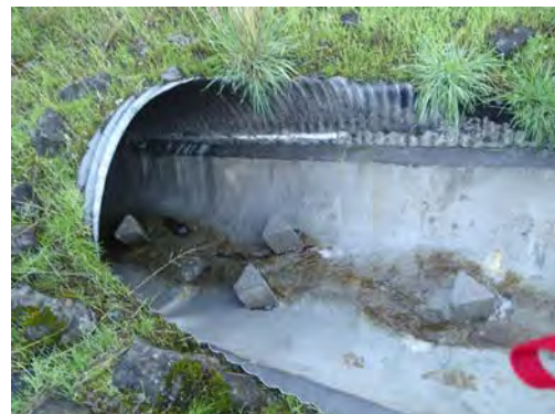
Roughness features creating turbulence, increased water depth, and longer flow path during low flow (10/26/16)
