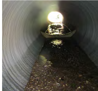
Inside culvert showing some accumulation of substrate near inlet
