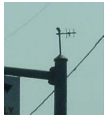
Wireless communications example: a radio antenna installed on a signal pole to enable remote communications to the intersection
