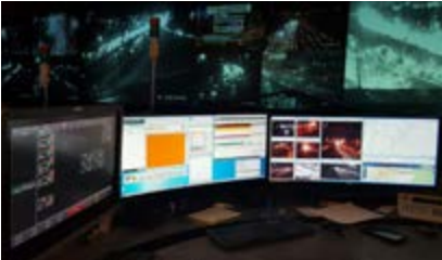
Transportation Operations Center
