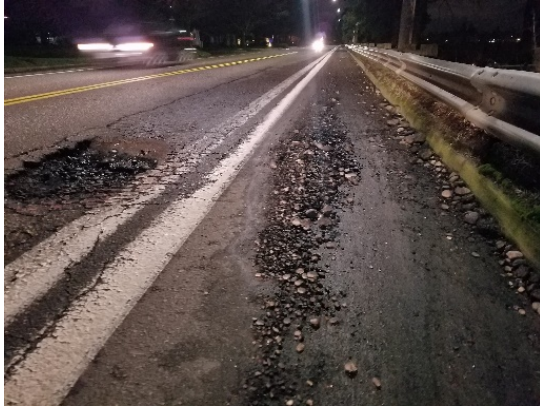
Figure 12: Poor rating, cracked pavement.
