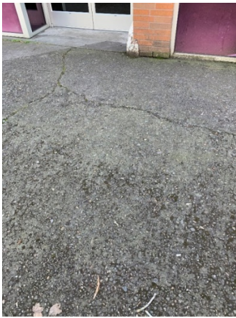
Figure 22: Example of Poor (P) sidewalk surface.
