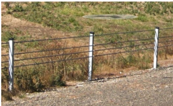
Figure 58: 4-STRAND - Other high tension cable barrier with four cables not matching the description of either the CASS-S3-M10 or the BRIFEN O-Post systems shown above.
