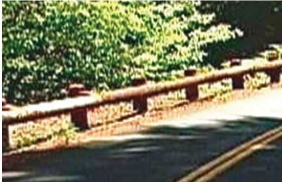
Figure 68: TIMBER (Round Timber) - The rail is made of round timber and has steel backing.
