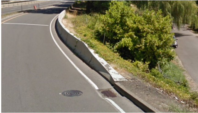
Figure 6: Sloped End Unburied - End slopes down toward the road.
