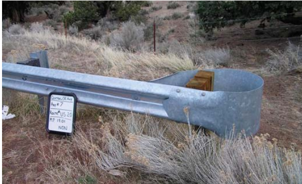
Figure 12: Blunt C Second post is not breakaway (see ET 2000).
