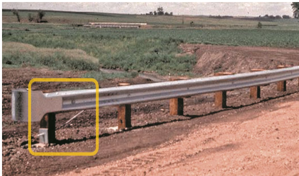
Figure 13: Breakaway Cable Terminal (BCT) - Terminal head has various forms. The first two posts are drilled to be breakaway (see ET 2000). A cable connects the back of the rail with the first post.
