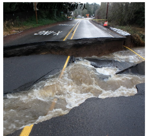
Figure 2: Ex. flooding and culvert failure during high intensity rainfall event (Hwy110 MP11,
