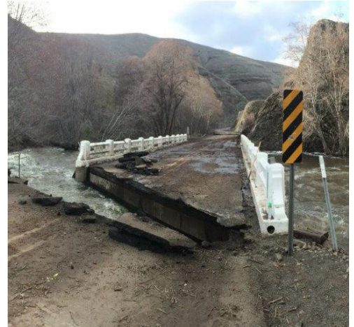
Figure 1: Ex. flooding impacting bridge (scour failure) during high intensity rainfall event (Rock
