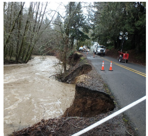
Figure 3: Ex. flooding impacting road during high intensity rainfall event (embankment,
