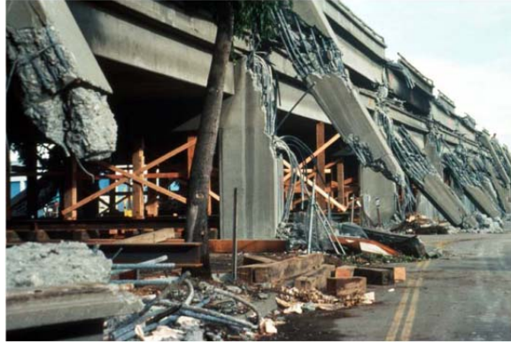
Figure 5.2: Collapsed Cypress street viaduct in Oakland during the 1989 Loma Prieta Earthquake ( USGS and Wilshire 1989 )
