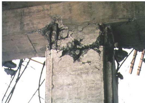
Figure 5.1: Poorly Confined Column in 1971 San Fernando Earthquake
