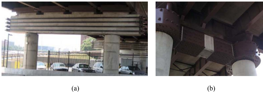
Figure 5.5: Retrofit measure for bent caps. (a) Posttensioned rods. (b) Steel Jackets. (Wright et al. 2011)
