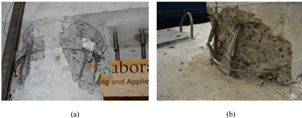
Figure 7.23: Damage on As-built RC bent. (a) Buckling of Steel, (b) Rupture of steel
