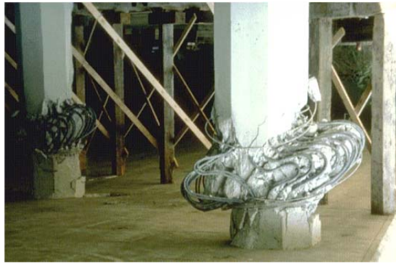
Figure 5.3: Damage in RC columns on the Simi Valley Freeway during the 1994 Northridge Earthquake ( Teng 1994 )
