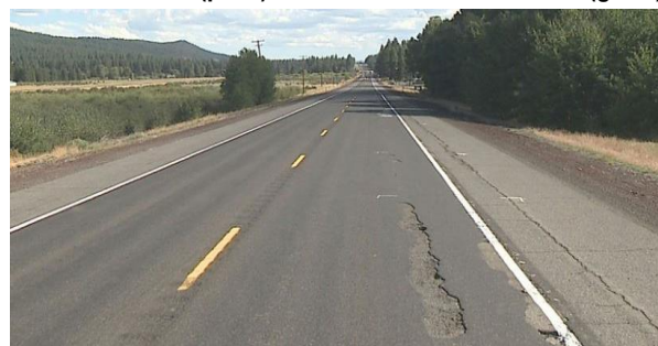
State – Potholes (poor) National – No rut or crack (good)
