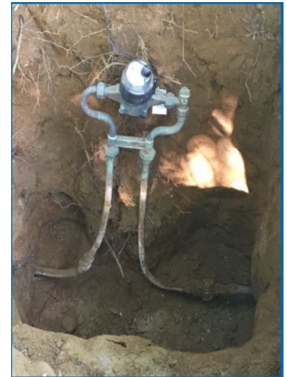
Example of Meter Pit Source: LSLR Collaborative 2018
