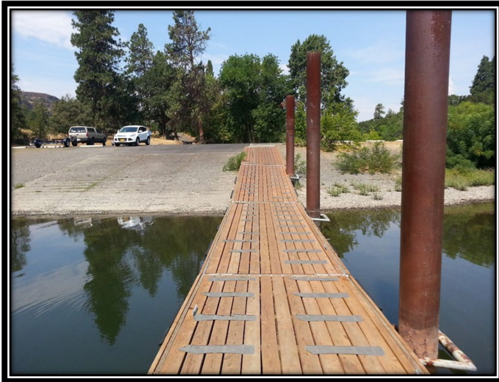
Figure 3 – Dock framework is rotted and in poor condition
