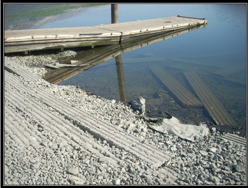
Figure 5 – Concrete planks are becoming disconnected creating hazards for watercraft launch and retrieval
