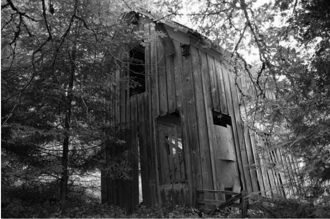
Figure 3.2.6 - Looking northeast at the William N. Ruble's House. The back half of the building is missing, and the structure could collapse at any moment. (author's collection)
