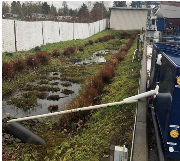
Constructed bio-swale for stormwater secondary treatment
