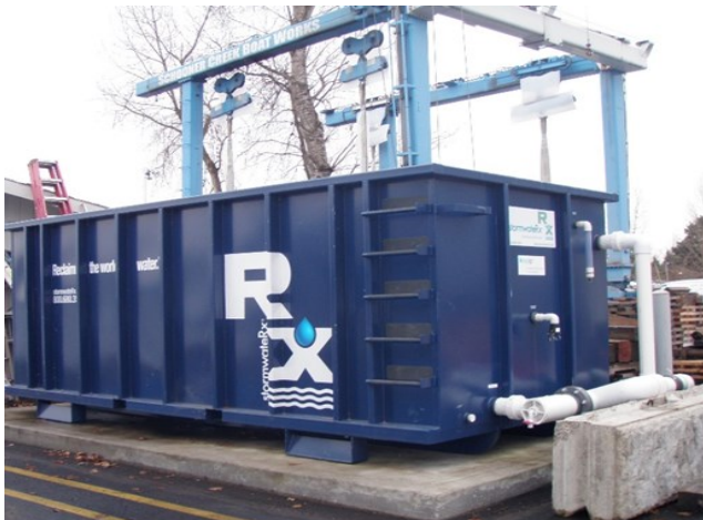
Primary stormwater treatment system (StormwaterRx)
