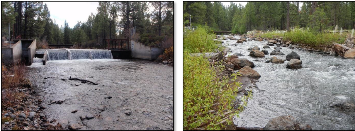
Figure 5-3. An irrigation diversion weir on Whychus Creek near Sisters, Oregon before (left) and after (right) the construction of a roughened channel.
