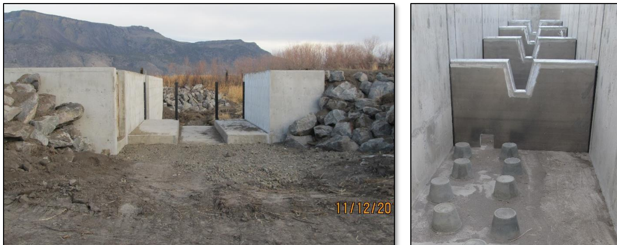
Figure 6-7. The reconstructed Rookery diversion weir on lower Honey Creek (left), includes wooden cross-walls, a 9-inch square orifice in each cross-wall, and artificial boulders on the ladder floor to reduce velocities (right).
