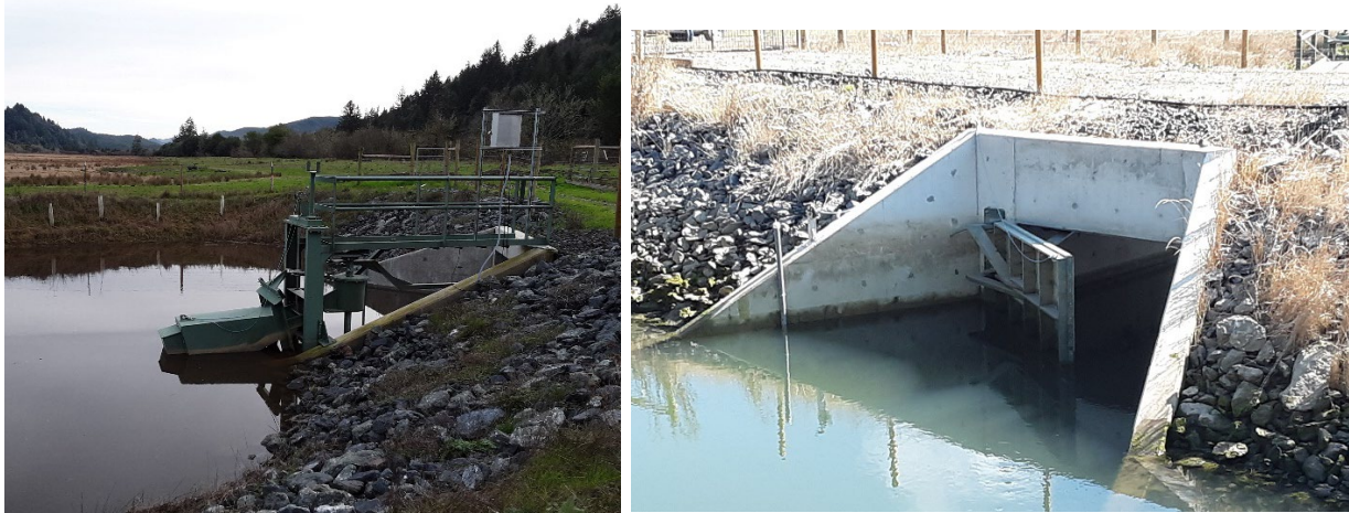
Figure 5. An 8'x8' aluminum side-hinged MTR tide gate was installed at the Seestrom project in 2019. The landward side of the MTR structure uses a counter weight to keep the tide gate door open during rising tides (left photo). The tide gate door is installed on the riverside of the concrete culvert (photo right).
