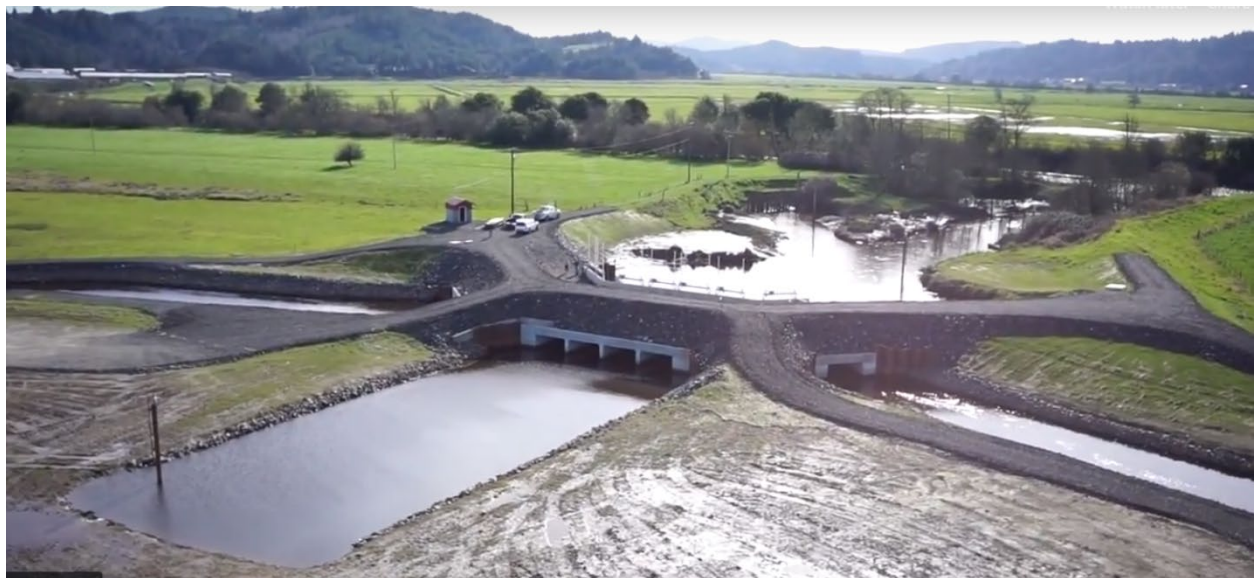
Figure 4. Aerial view of the landward side of the Winter Lake tide gate structures during construction phase.
