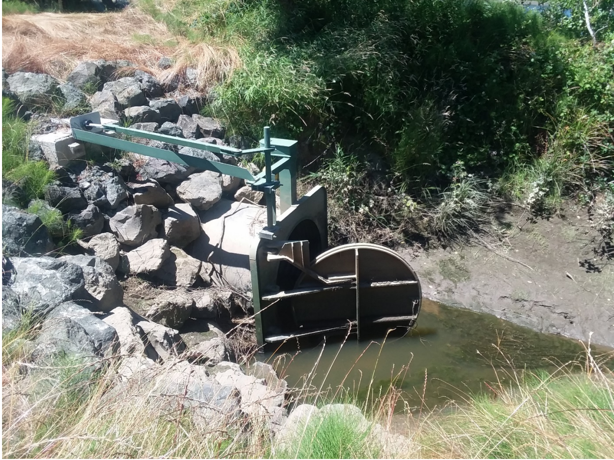
Figure 2. A 6' diameter aluminum side-hinged MTR tide gate was installed at the Cochran project in 2017. The tide gate door is installed on the riverside of the culvert.
