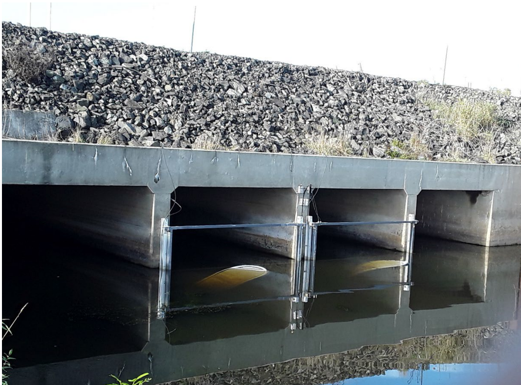
Figure 6. Winter Lake Unit 2 PIT antenna array on tide gate culvert 2B and 2C. The pass thru (gray fiberglass structure) and sail (white sail in water) antenna are installed on the landward (upstream) side of the tide gate culvert whereas the tide gate doors are installed on the river (downstream) side of the tide gate culvert.
