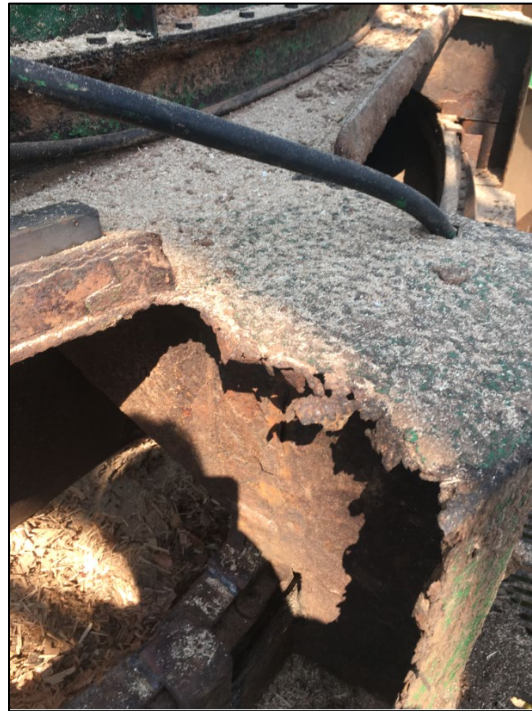
Figure 5-1: Steel Degradation at PWL Due to Exposure
