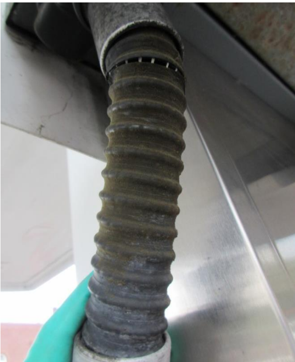
Balance Whip Hose- Torn
