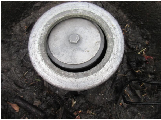
Poppet valve not sealing.
