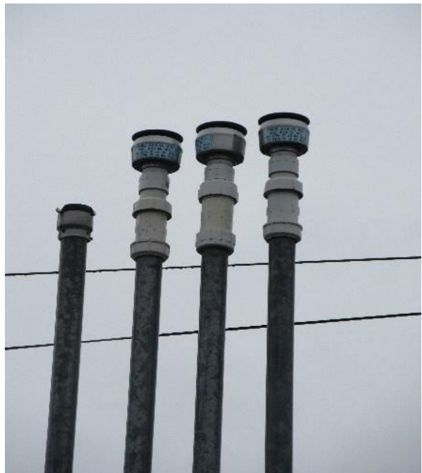
This picture shows three PV valves, one for each gasoline tank on site, and one open atmospheric vent (left) piped to the diesel tank. Note that one PV valve is acceptable for multiple gasoline tanks if the piping is manifolded together. All Stage II permitted sites require PV valves for gasoline storage tanks.
