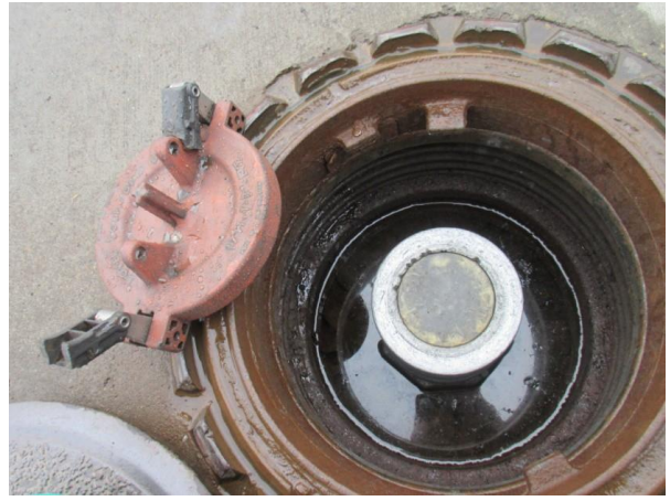
Dust Cap- Broken
