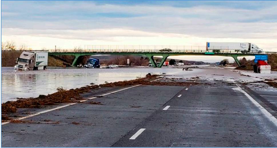
Flooding along Interstate 84 near Hermiston in February 2020. (Oregon State Police)
