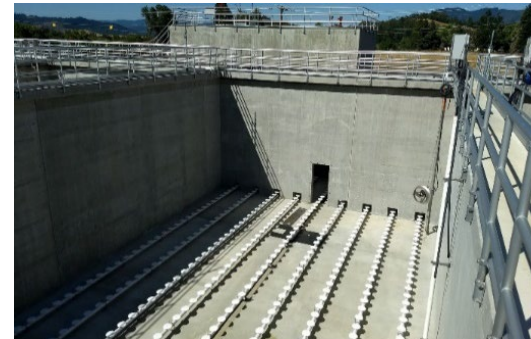
Wastewater aeration basin
