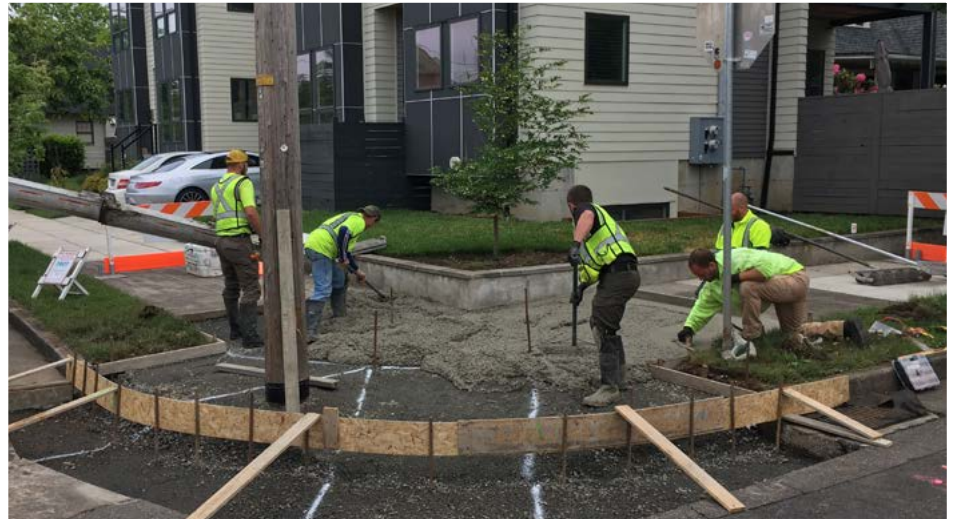
Workers at one of the Portland test sites moving wet, low carbon concrete.
