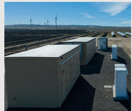
Wheatridge Facilities (PGE)
