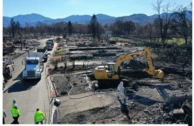
More than 5,000 structures were lost in the Labor Day 2020 wildfires.
